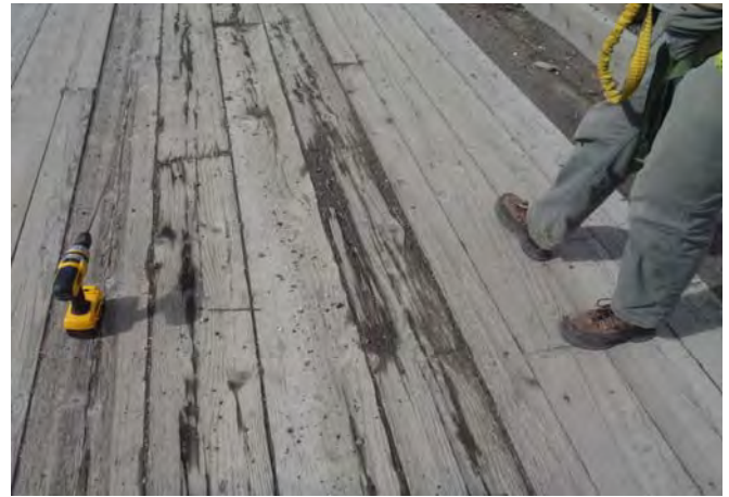
Figure 1-14: Pocket of rot in old planks, note condition of wearing planks.
