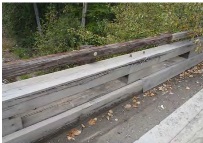
Figure 1-10: Downstream curb rail condition, note rub damage.
