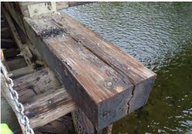
Figure 1-29: Pier 2 woods end cap, downstream end split.
