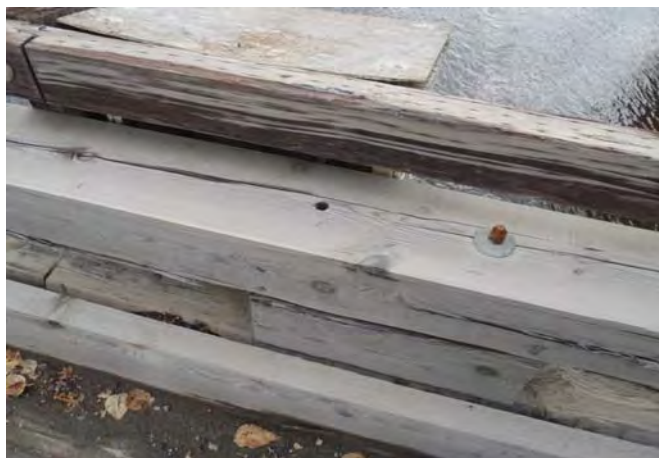
Figure 1-11: Typical missing curb rail anchor bolt.
