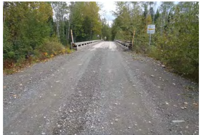
Figure 1-6: Looking towards woods end, note no delineators.
