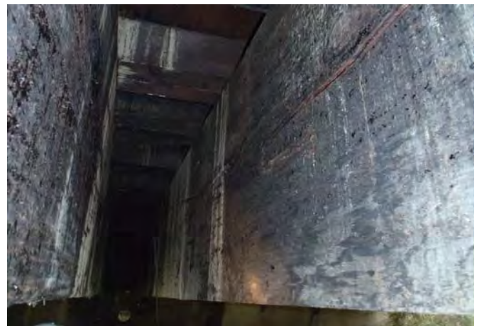
Figure 1-16: Span 1, typical interior stringer condition, stringer 5 downstream face shown.
