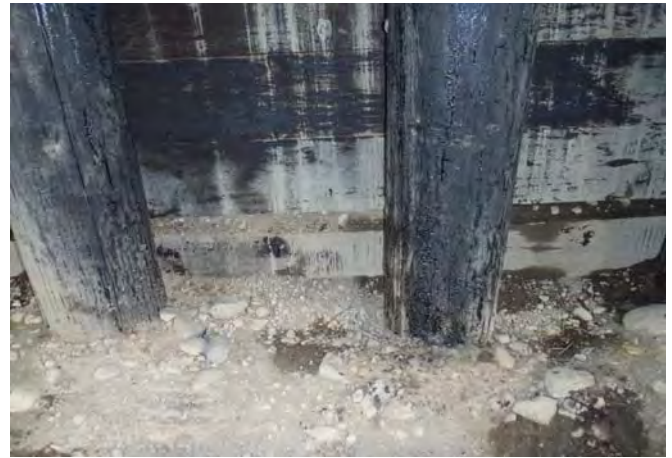
Figure 1-26: Woods end abutment ballast wall, gap between planks and minor scour.
