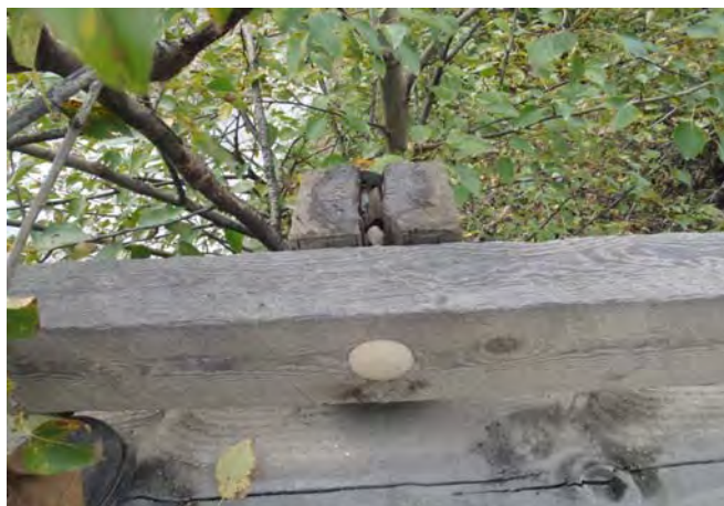
Figure 1-12: Typical end split in downstream hand rail.
