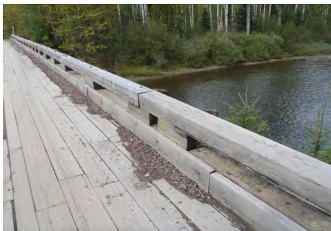
Figure 1-9: Upstream curb rail condition.
