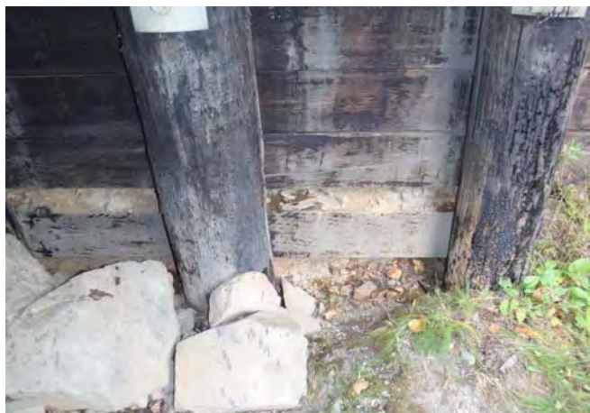
Figure 1-24: Camp end abutment ballast wall, gap between planks and sign of scour.
